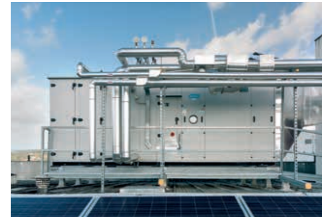
Figure 23: Example of an outdoor installation
