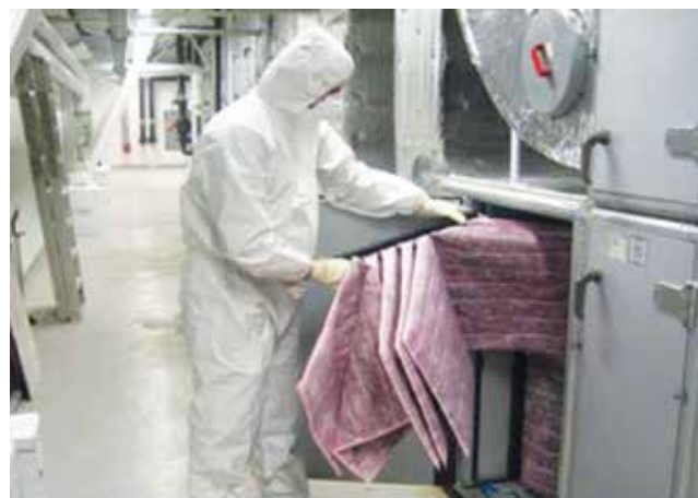
Figure 9: Personal protection equipment for filter replacement
